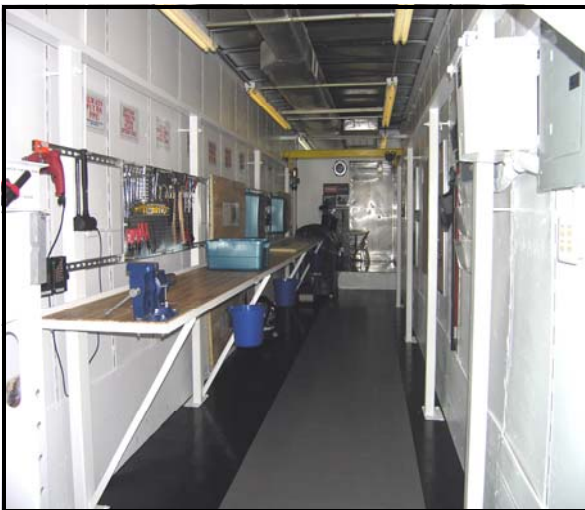
Mobile Centers Facilitate Requirements for Clean and Contaminated Valves and Components
